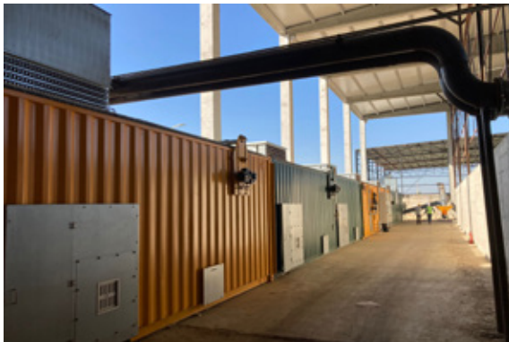
Reference facility: Turkey, 2022 RDF drying / 7.500 kg/h
